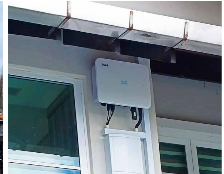
12kW Solar System in Malaysia (XG12KTR)
