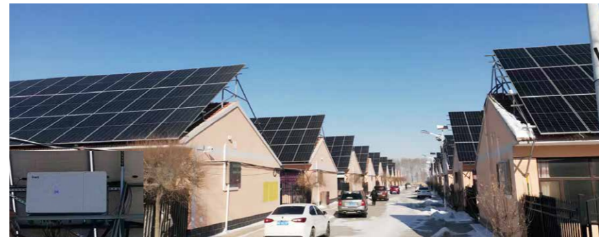
11.6MW Rooftop PV Plant in Hebei, China (XG110KTR, XG60KTR)
