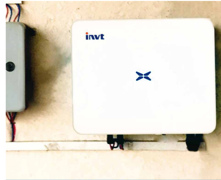
10kW Solar System in Armenia (XG10KTR)
