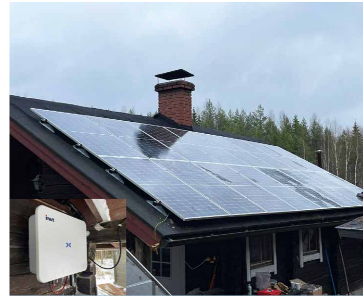
8kW Solar System in Finland (XG8KTR)
