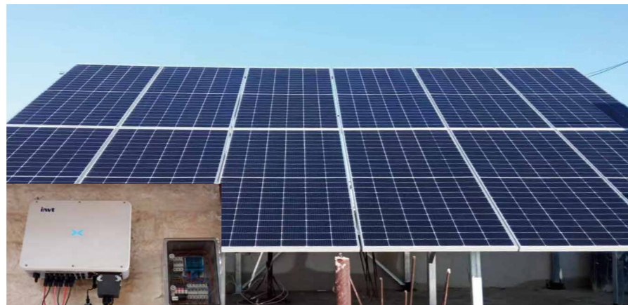
30kW Solar System in Israel (XG30KTR)
