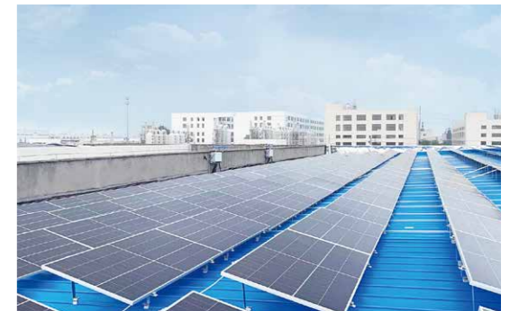
125kW Rooftop PV Plant in Slovakia (XG50KTR, XG25KTR)
