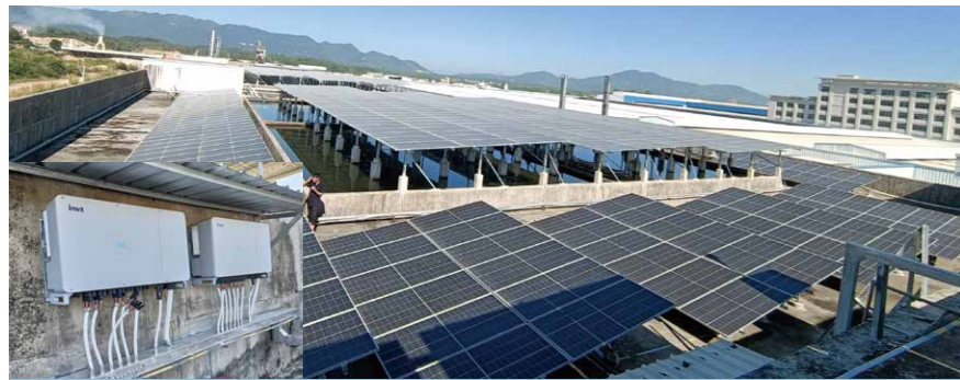
2.4MW Rooftop PV Plant in Guangdong, China (XG136KTR-X)
